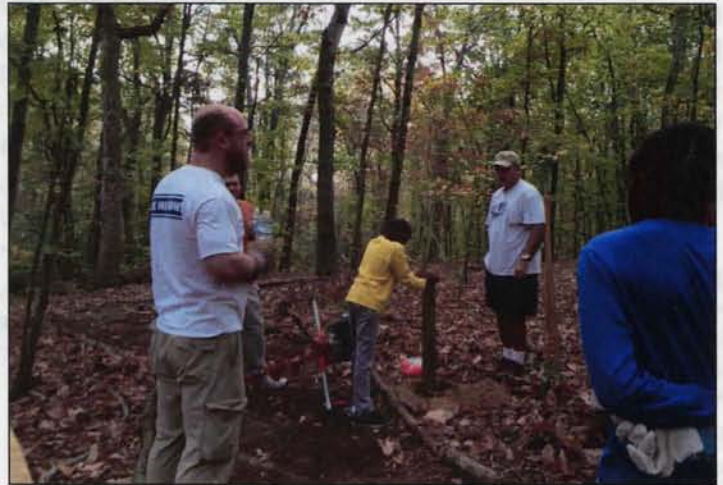
Bart Foster, Lionel and Jalon Blake, Berry Walton, and Patrick Simmons work on setting a post along the reading trail at Friendship Elementary School.
